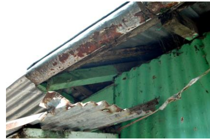
Decaying timber and corrugated roofing
