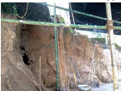
Hole found under the existing toilet block
