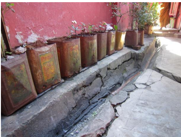
More cracks appear as the land moves.
