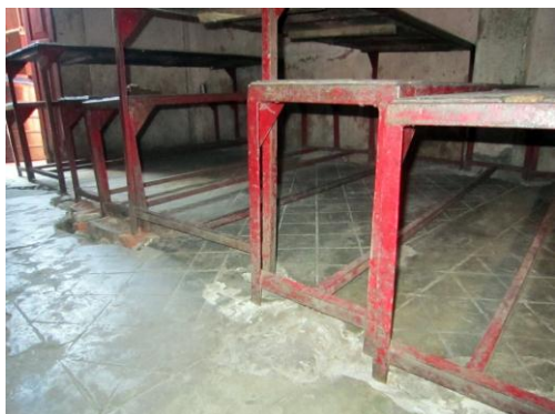
Concrete fill in the floor of the dining room which split open
