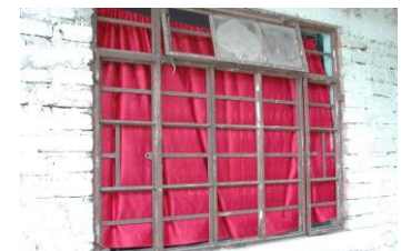
Another problem - lack of window glass
