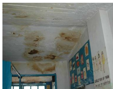
Water stains in the ceiling
