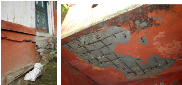
Cracks are evident and cement render is falling off at the boys' orphanage
