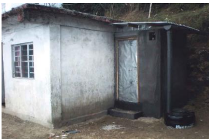
The new toilet at Agam Singh school. The water tank has now been removed and will be relocated.
