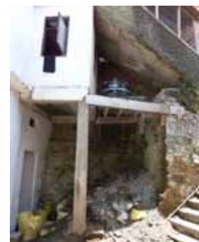
Water harvesting tank
